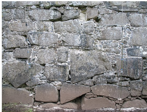
Fig. 2 The walls of the cathedral is made of irregular basalt boulders. The cavities in between are filled with smaller pieces of rock held in place by the mortar. Test area for restoration on the north side of the north wall
