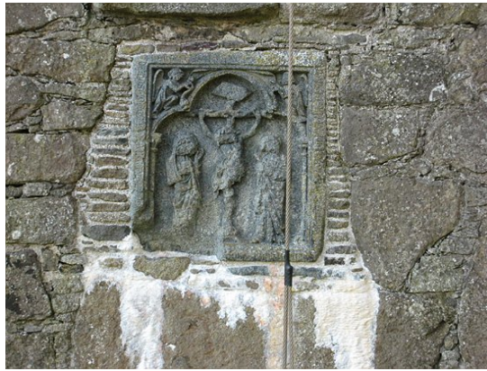
Fig. 5 The lime deposit below the relief on the east wall has leaked from the lime mortar used for the joints.
